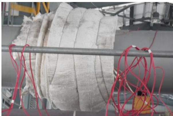
Fig.18: Insulation around the joint
