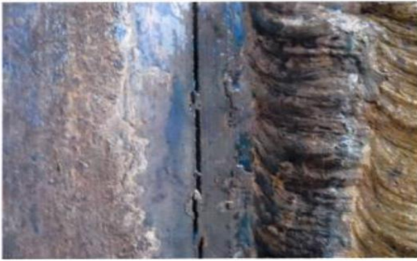
Fig.8: Crack on the flange-neck
