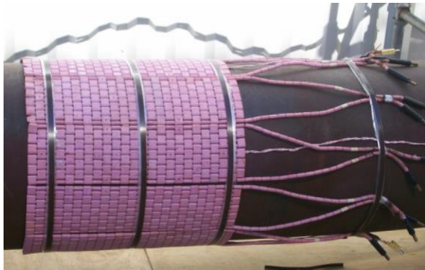
Fig.17: Induction heater arrangement for Local PWHT
